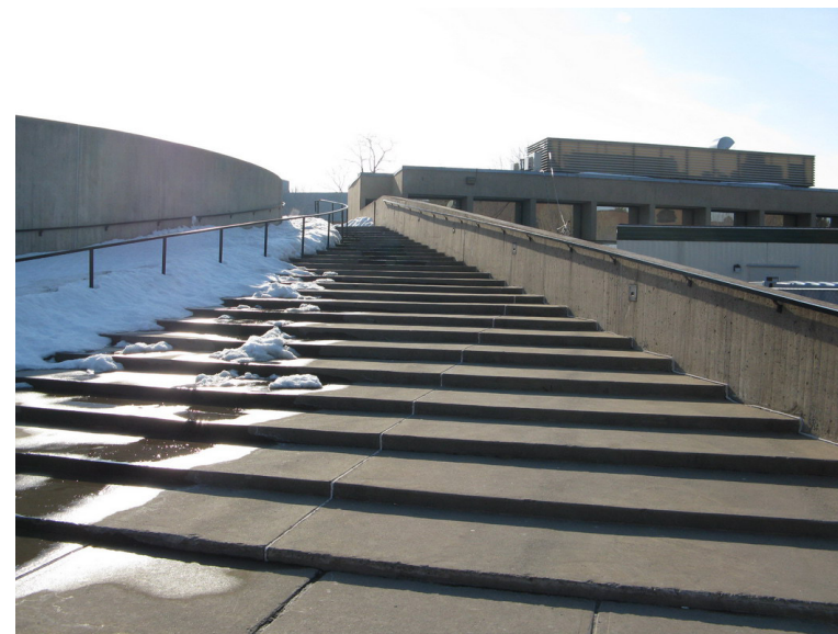
Long flights of stairs at the Library are a barrier to universal site accessibility. An alternate path exists, but it is not well marked.
