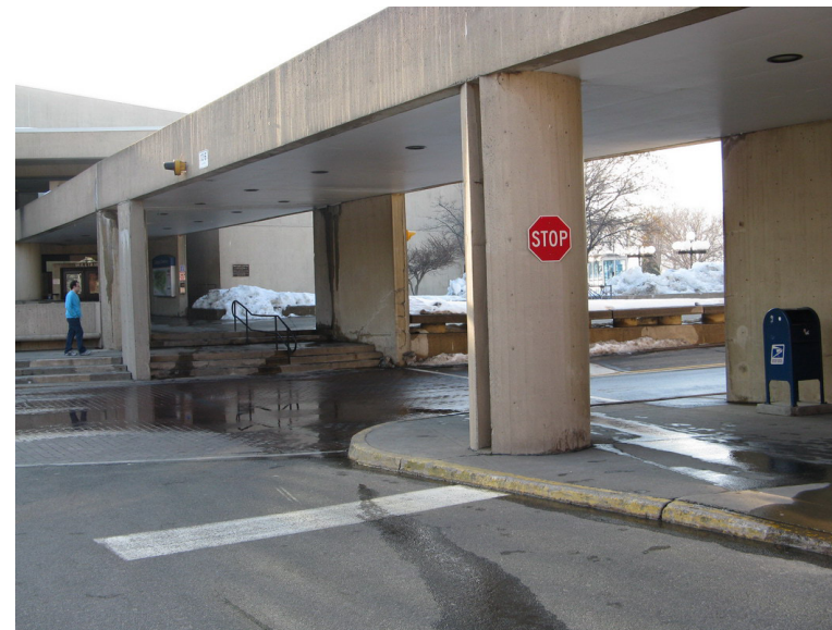
The crosswalk and Williams Center entrance lack direct accessibility from the Spine walkway.
